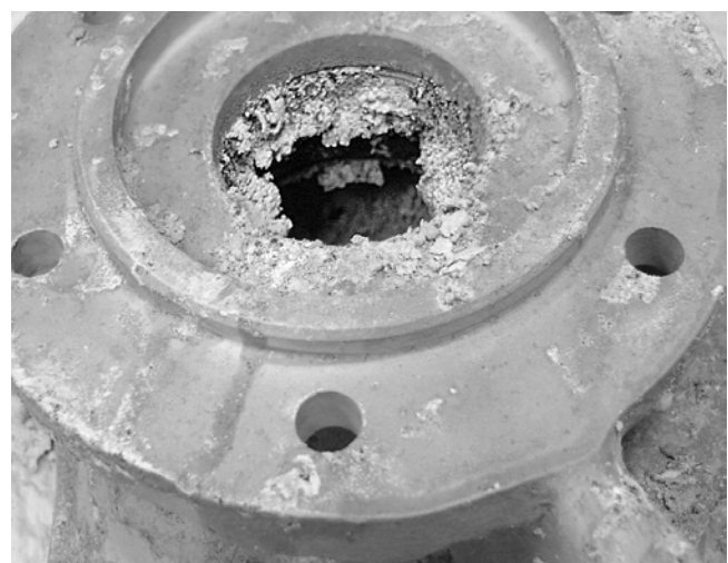
Figure 3-24. Magnesium Corrosion Products
